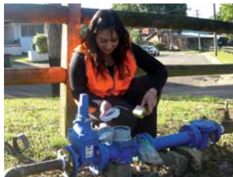
Rafaah Mian, Council's Student Engineer checks the reading on a water saving device
